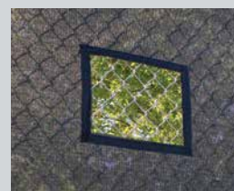
Reinforced Air Vents
